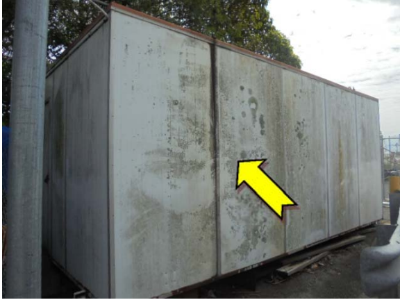
Photo Exterior, throughout, walls – suspected 1. lead-containing white upper paint system.
